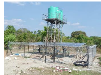
Water tanks with security fence and solar panels
